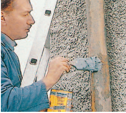
Rusted drainpipe: small cracks are bridged thanks to fibres.
