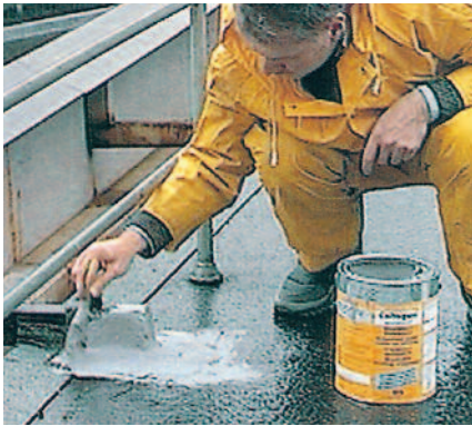
Repair leaky bitumen coatings at minimal cost.
